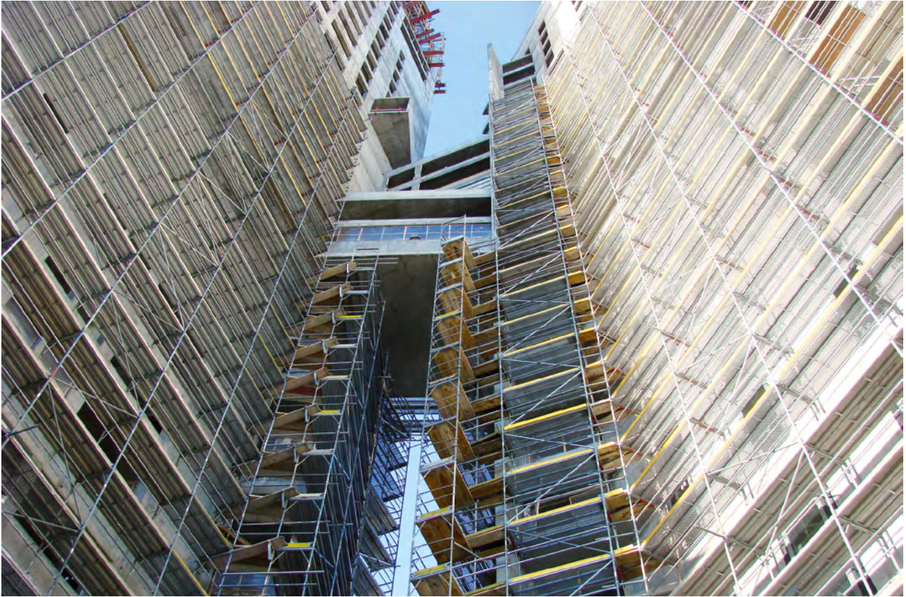
▶ High up – also the standard design is applicable for heights up to 24 m
