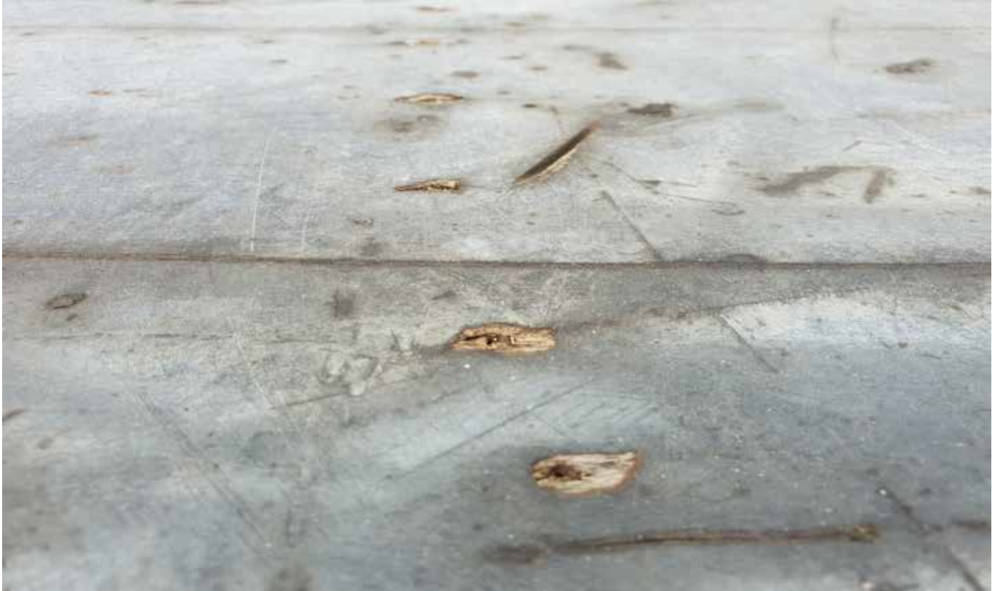
Photo1 Example photograph of a damage
