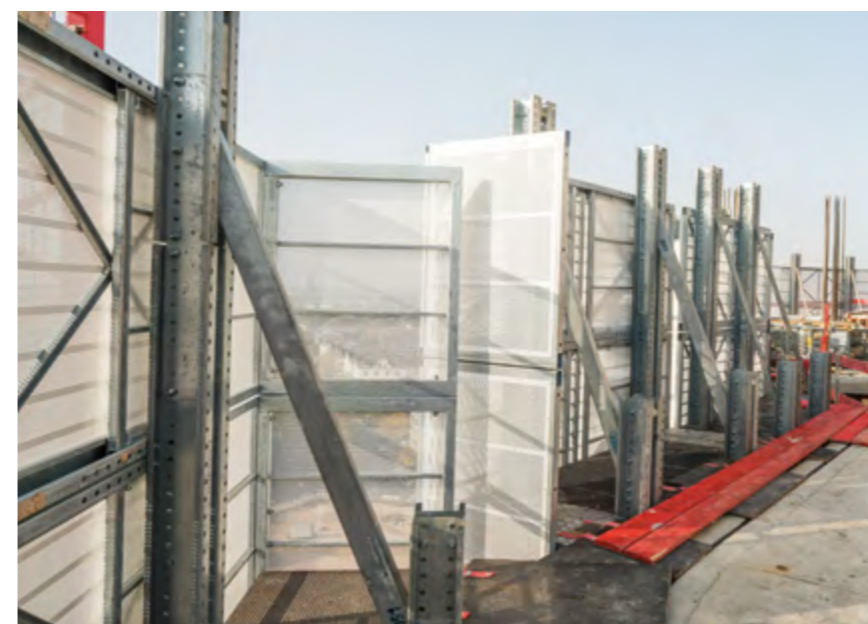
▶ Improved on-site and public safety due to full enclosure of the working environment
