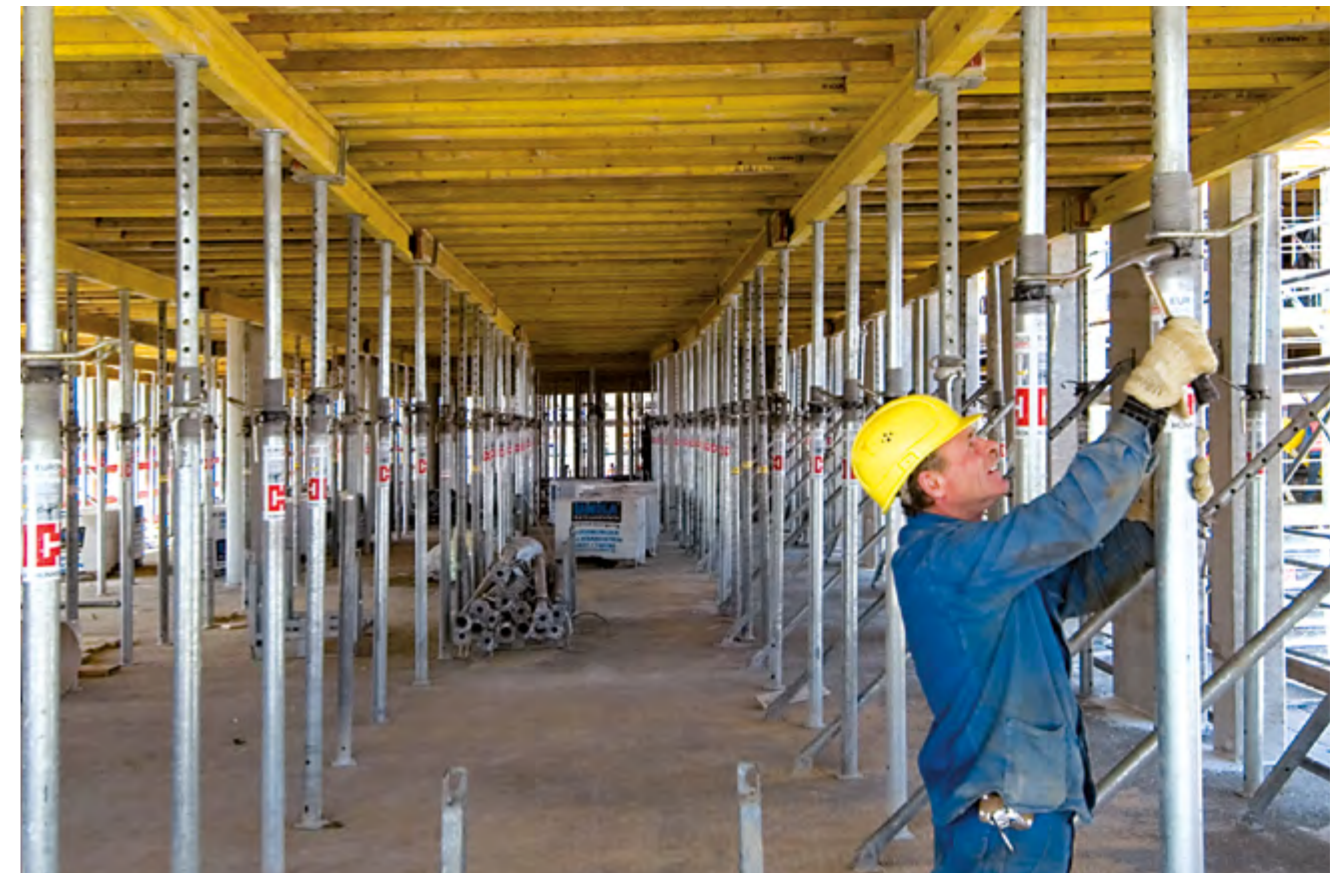
▶ Stripping is made easier by lowering the forming plane by about 6 cm using the adjustment nut of the steel props
