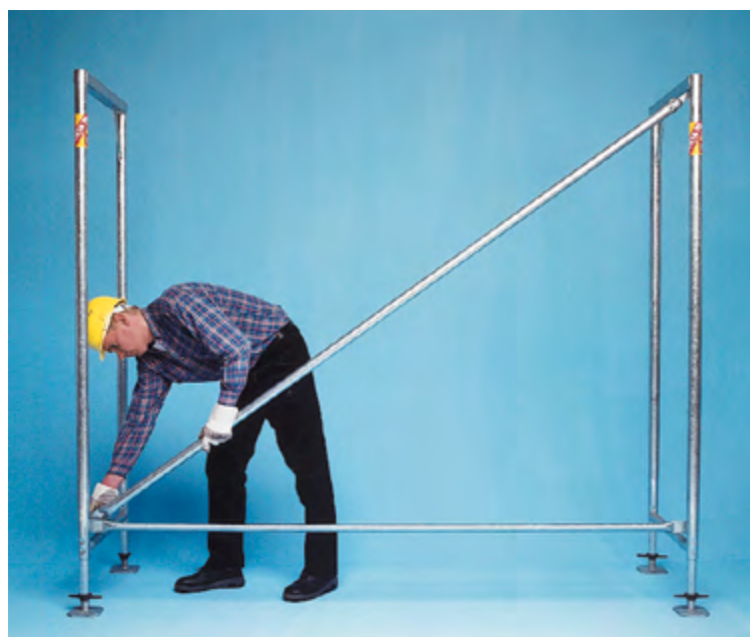
▶ Safe and inevitably plumb-vertical erection already after assembly of the first bay
