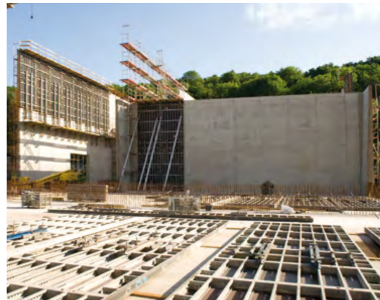
▶ By using facade soldiers, the 16.73 m high walls of a terminal were shuttered in two pouring cycles instead of three.
