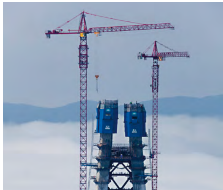
► Upwards and higher: forming operations at heights of over 300 m are no challenge for SCF
