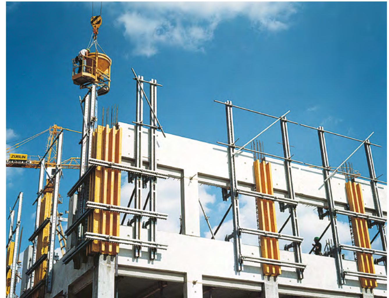
▶ The facade formwork enables mixed structures to be formed in economical procedures.
