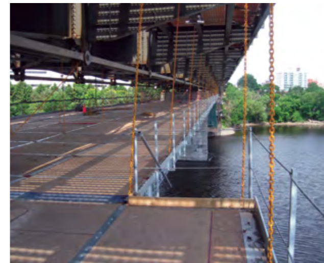
► QuikDeck provides safe and spacious work platforms for new constructions, refurbishment and repair work
