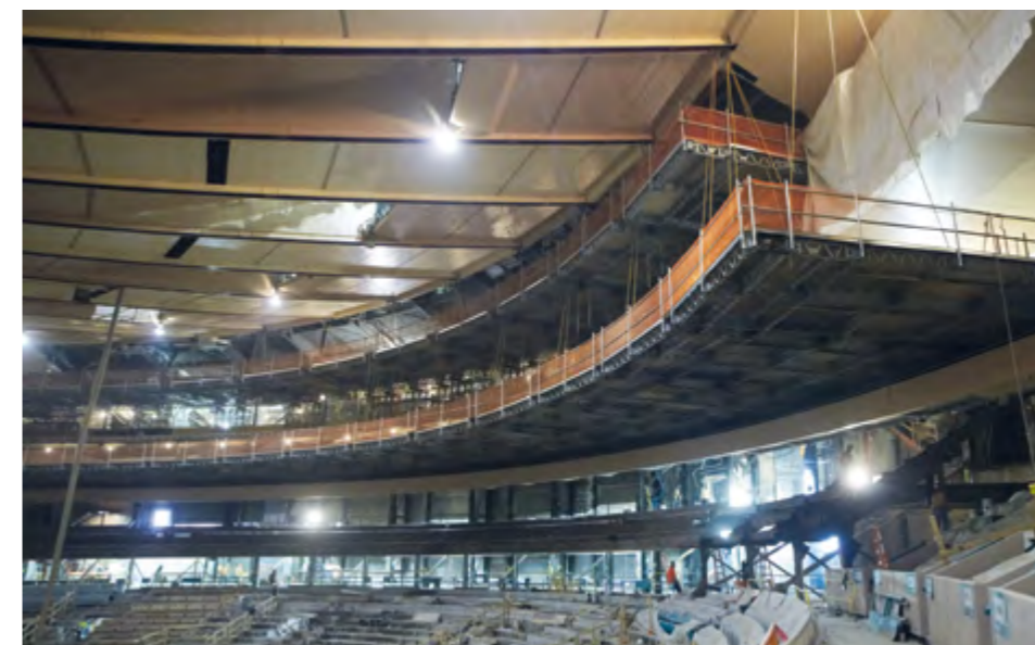
▶ Madison Square Garden (New York City) During renovation work in Madison Square Garden, Penn Station, which is located underneath and serves as a major transportation hub in New York, had to remain open. QuikDeck was the perfect solution for worker access
