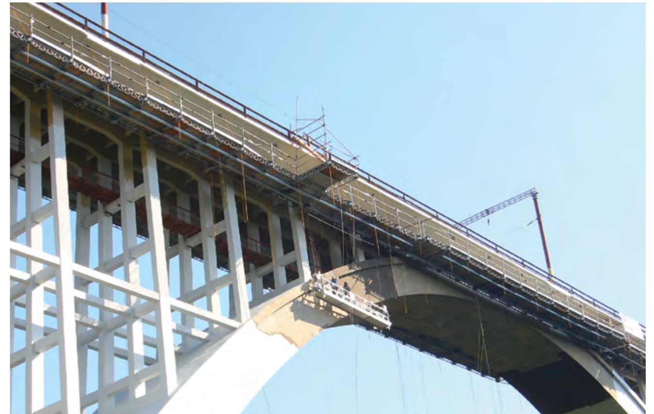
▶ The QuikDeck platforms suspended from the Romanian railway bridge of Caracău Viaduct provide a consistent, safe working level and replace classic spatial scaffolding. This lowers the costs of bridge maintenance and speeds up the work
