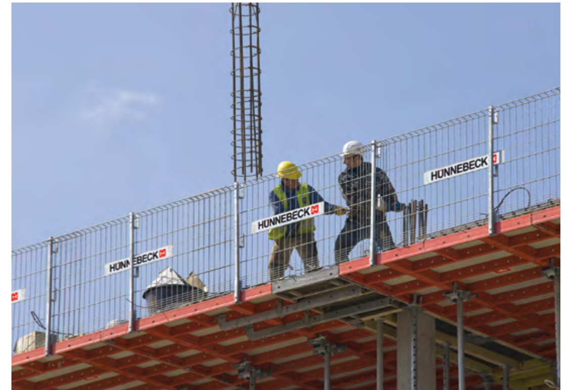
▶ PROTECTO is compatible with all Hünnebeck slab formwork systems, such as TOPMAX as shown here
