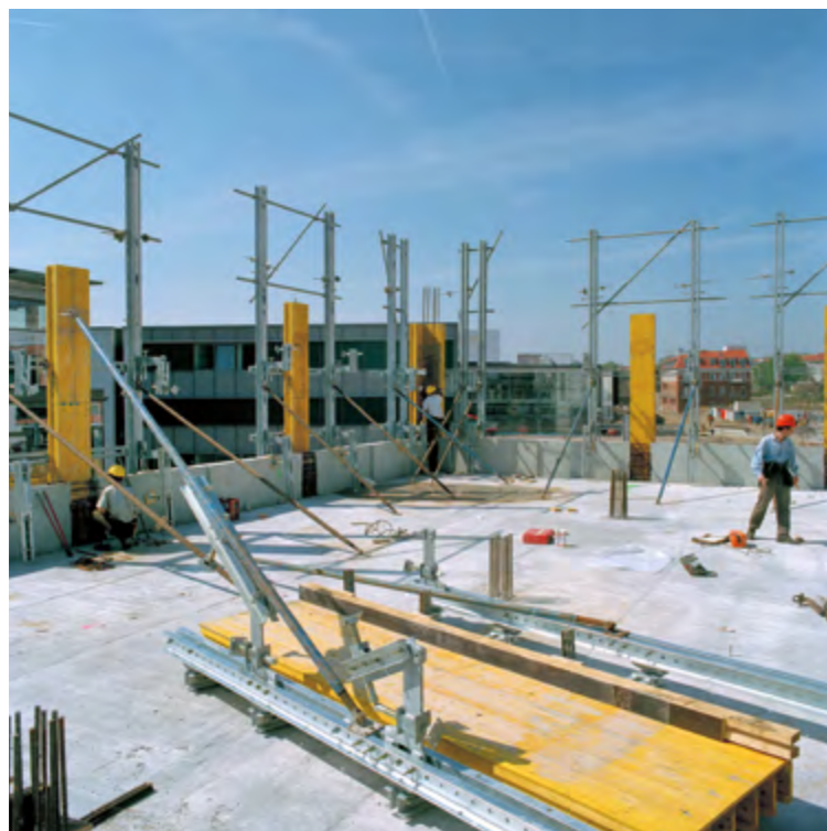
▶ Low quantities of equipment kept on site thanks to leading construction cycles
